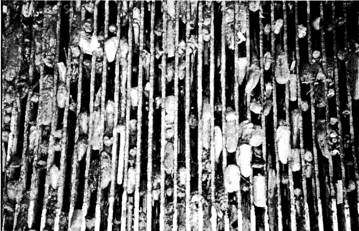
Photo 5. Debris Clogged Fish Unit Trash Rack
